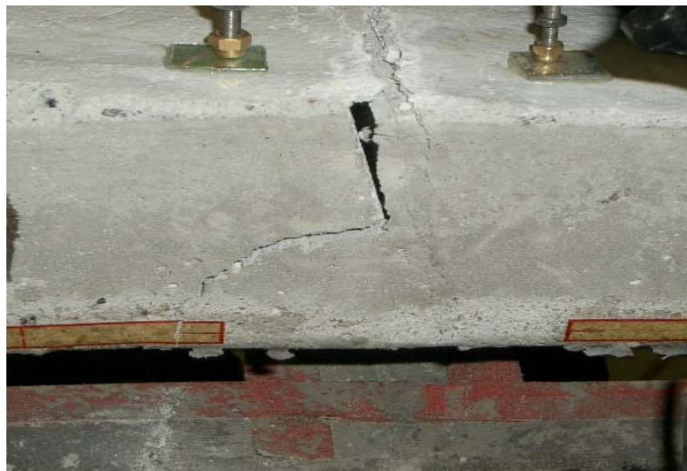
Fig 6 Crack occurred at the shape edge of aluminium Joiner
