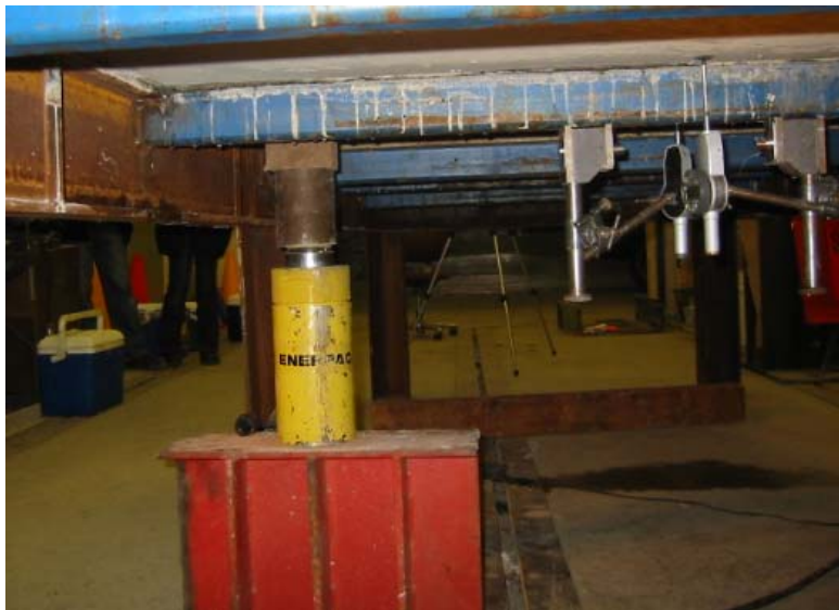
Figure 6. Slab 2 being pushed up at a corner
